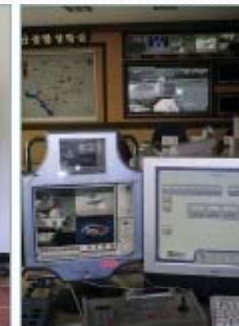
Integrated Monitoring System
