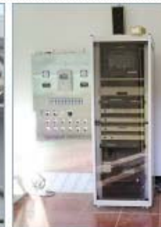
Remote Control System
